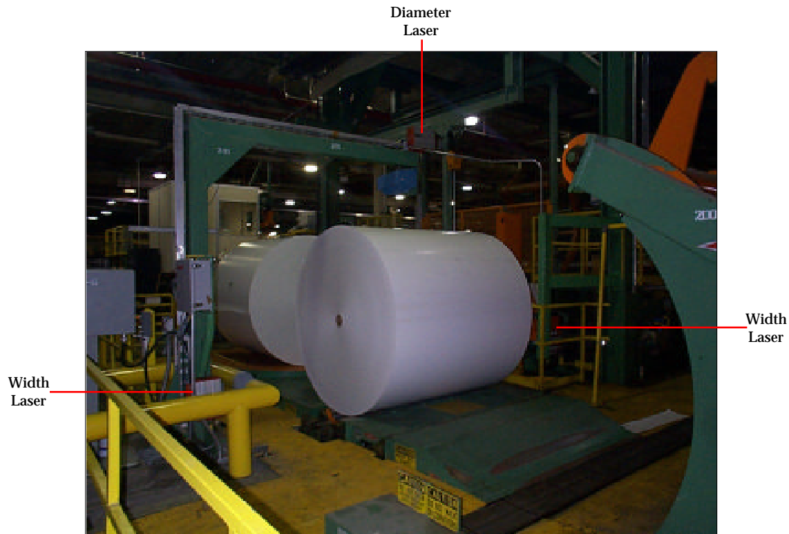
Picture above is a typical Paper Mill. There are three 3000 Series DSP sensors measuring the diameter and width of the paper rolls. The two sensors looking at the ends are measuring the width while the one above measures the diameter.
